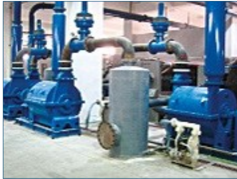
Vacuum pumps of washing unit
