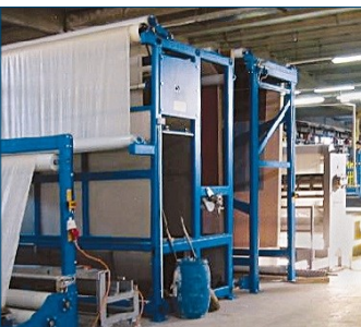
Unrolling, J-box, lint removal, pre-steamer, edge guiding and pull roller
